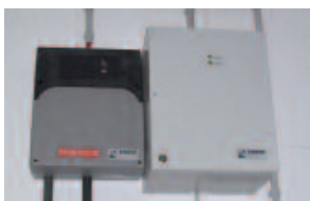
... the aspirating smoke detection system ...
